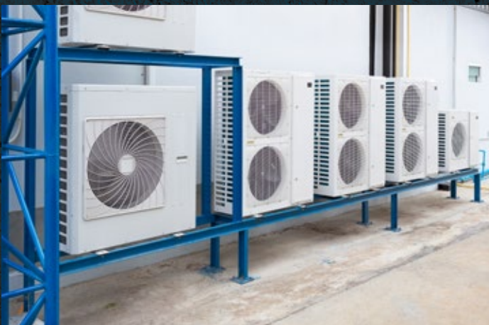
REFRIGERATED AIR HANDLER / CONDENSING UNITS
