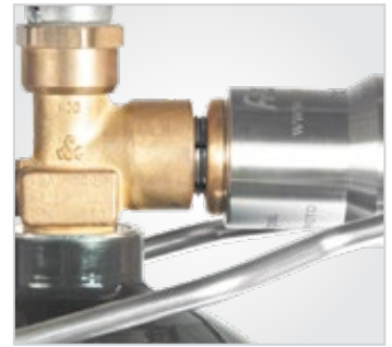
Figure 7d. Exposed threads indicating possible short connection with internally threaded cylinder valve.
